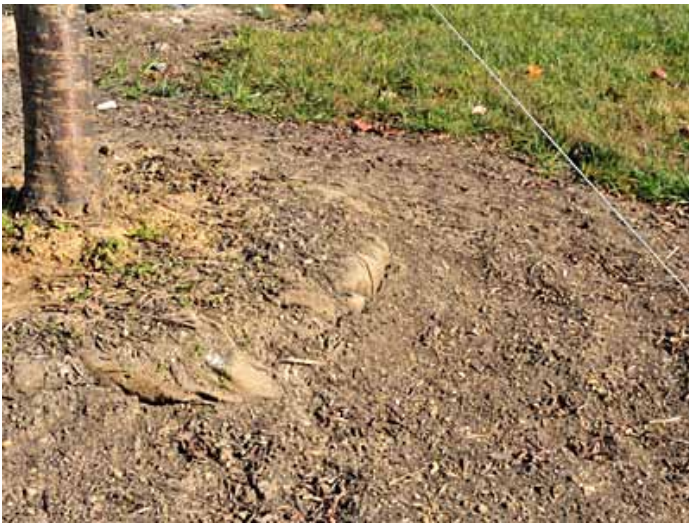
Soil and mulch washed out due to improper grading.
