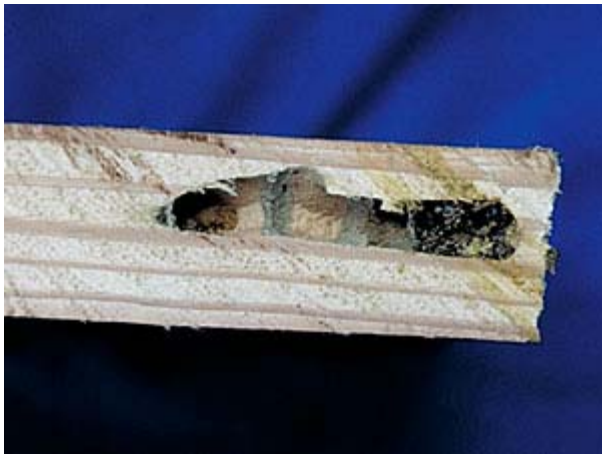
Carpenter Bee Tunnel
